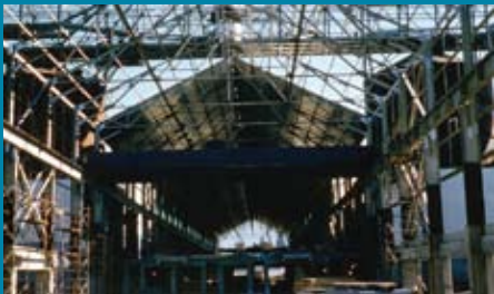
The skeleton of a potroom from below.
